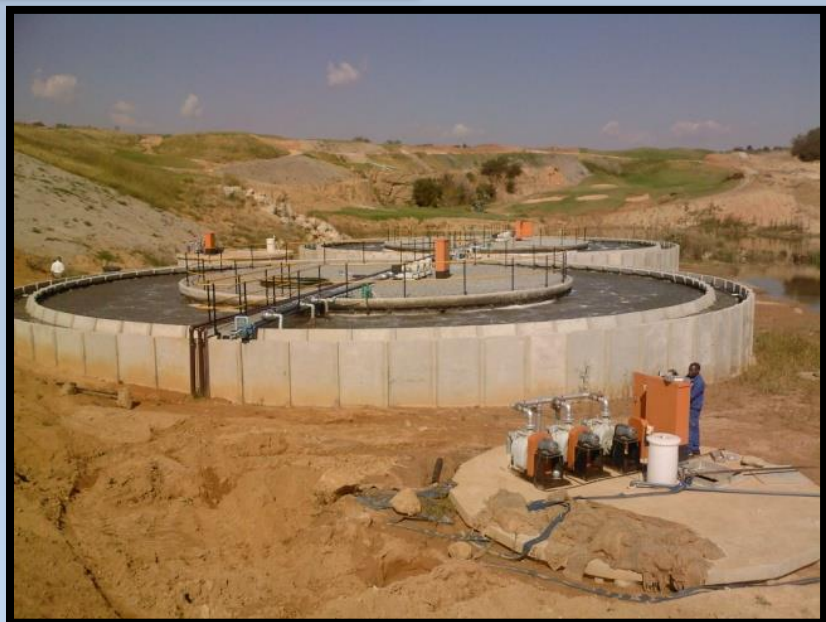
Concrete Sewage Plant Johannesburg 1.2ML/day
